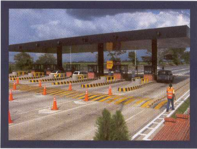
IRD Toll System installed for Unión Temporal Vial del Valle del Cauca y Cauca near Cali, Colombia.
