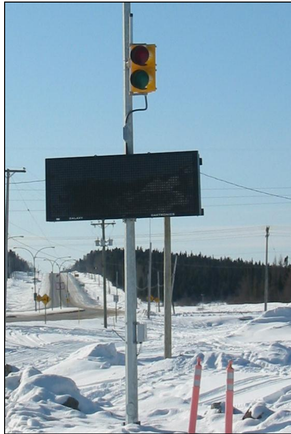
Figure 5 Changeable Message Sign and Red/Green Signal at Inspection Station
