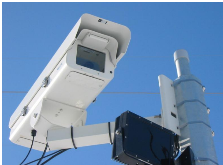
Figure 2 Side Fire Camera System
