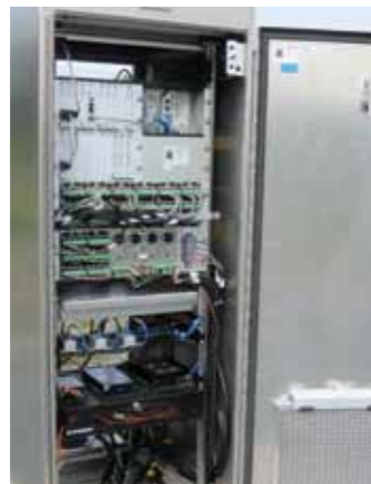
A weatherproof cabinet houses the iSINC
