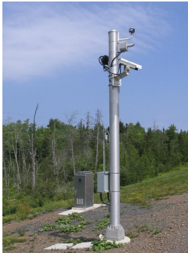
Figure 3 – Camera, Overheight Sensor and Electronics Cabinet, Deerwood NB
