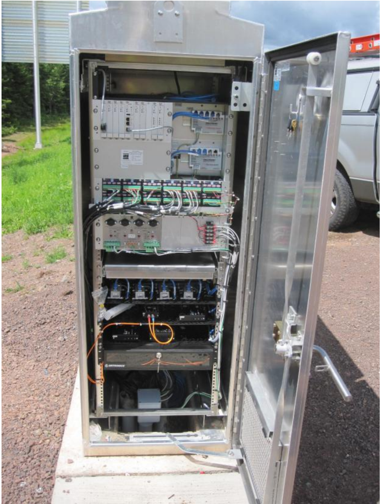
Figure 4 – iSINC WIM Electronics Cabinet – Salisbury, New Brunswick
